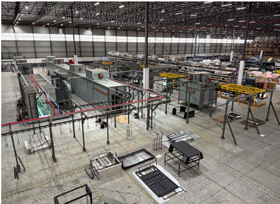
“The next big thing for us has been the design and commissioning of our new powder coating plant. It has been custom-made and installed by Bendet Engineering Services. It features both an automated facility as well as a manual facility where we can run different kinds of batch runs. Previously with our powder coating facility – we’ve long done powder coating in-house – we had to run two shifts. That will now consolidate into one shift.”
